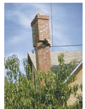
This chimney broke and nearly fell in the 1969 magnitude 5.6 Santa Rosa earthquake (photo courtesy NISEE).
