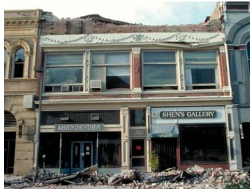
These small businesses in Santa Cruz, California, were heavily damaged in the 1989 magnitude 6.9 Loma Prieta earthquake, but both eventually reopened (USGS photo).
