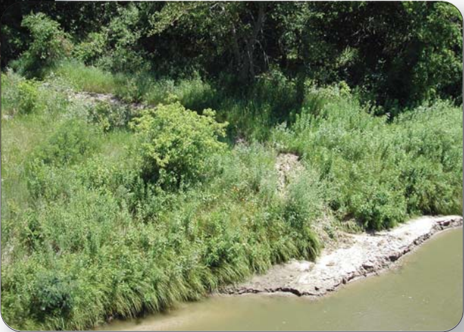
Sand transport after a storm from bank near bridge crossing where roadway construction disturbed existing grasses.
