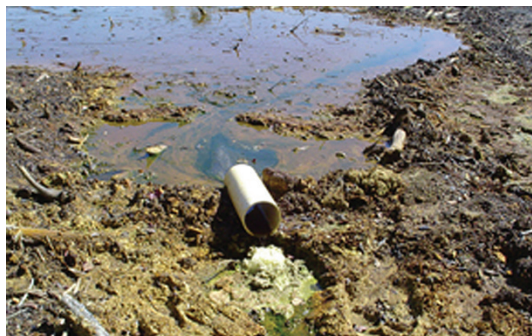
Photo 2. Seep at the Rehoboth reclamation site.
